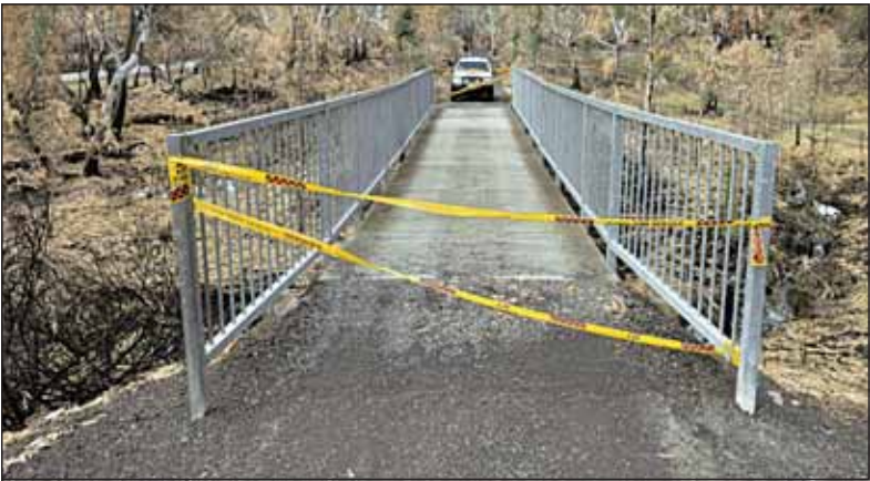
The bridge at Kanumbra provides an example of the damage caused by the January 2026 fires, and why the rail trail remains closed in many locations. -S
