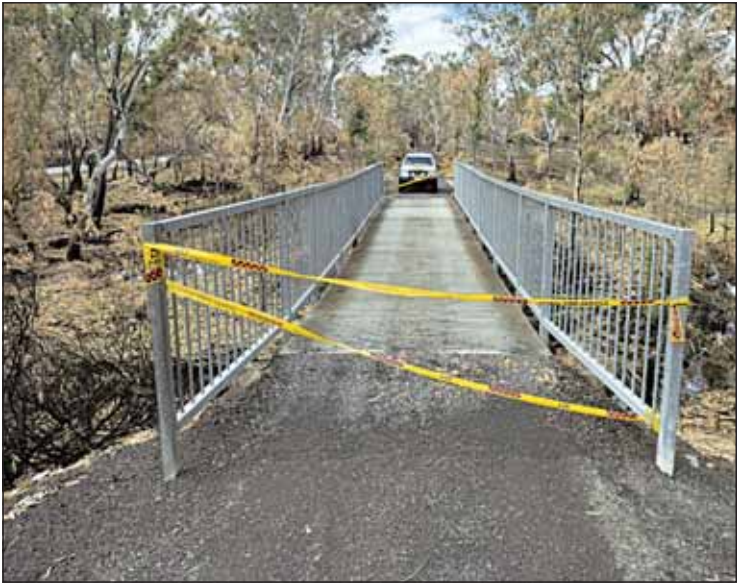
The bridge at Kanumbra provides an example of the damage caused by the January 2026 fires, and why the rail trail remains closed in many locations. -S
